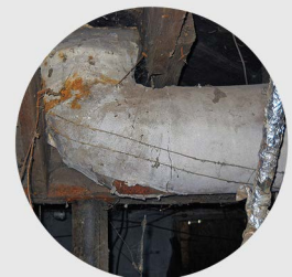
Heating System Insulation
